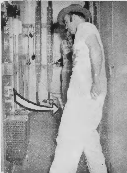
First step in the cutover was Adolph Arends pulling the main fuse (see arrow); this "killed" the old exchange for the first time since it was installed about 1934.
